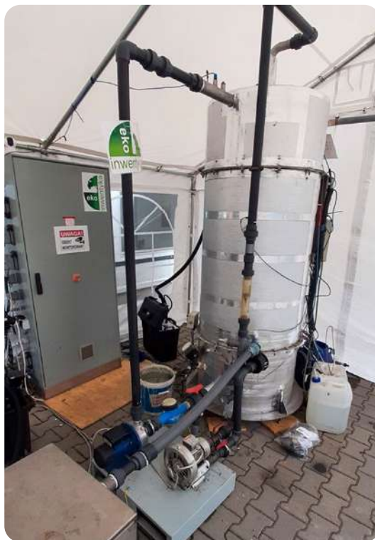
The Texen POLAND pilot biotreatment facility
