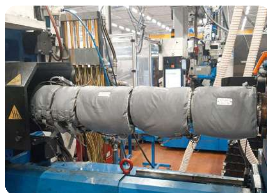
Insulating sleeves on an injection press at Texen CMSI
