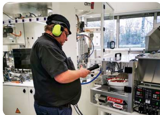
Detection of leaks at the Texen CMSI site
